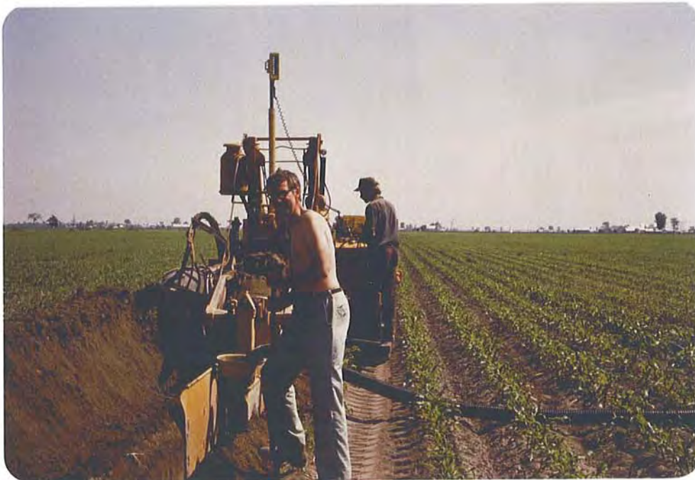
Greg Bostock and Drainage Richelieu trencher operator installing polyethylene pipe to retrofit a Charbonneau tile drainage system for Controlled Drainage and Subirrigation in 1982.
